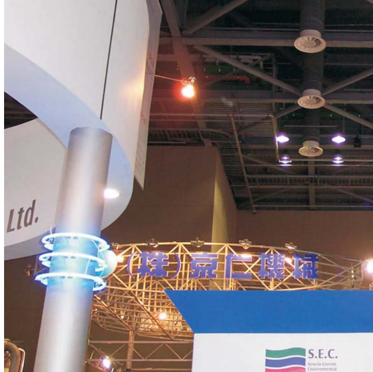
Radial outlet, type RA-V2, at Kintex Fairgrounds, Goyang City / ROK
