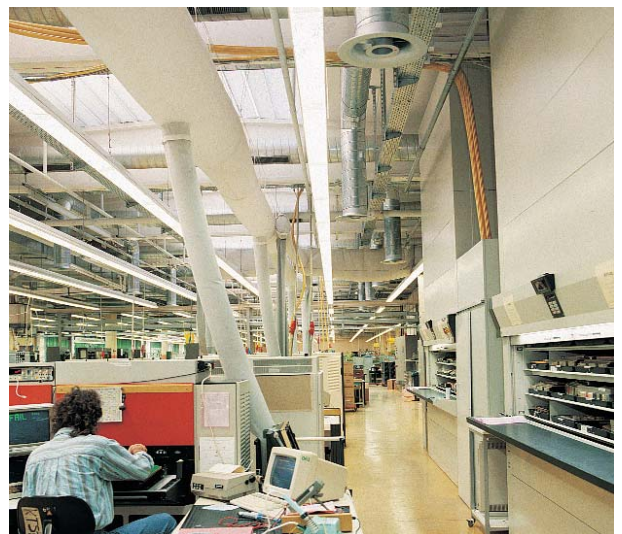
Variable twist outlet with core tube, type DD-VK, in a production hall at Alcatel SEL, Gunzenhausen / D
