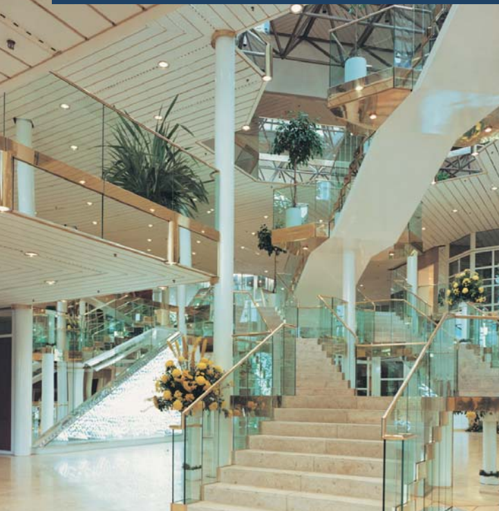
Induction outlet with fixed discharge direction, type IN-N, in the entrance hall of the Casino Hohensyburg at Dortmund / D
