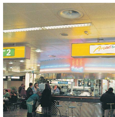
Twist outlet, type DD-N, in a terminal at the Vienna Airport / A
