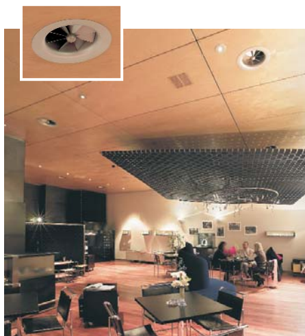
Twist outlet, type DD-N, in the canteen at 'Swarovski Kristallwelten', Wattens / A
