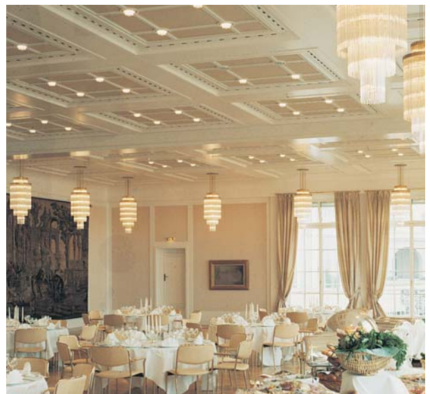
Induction outlet with fixed discharge direction, type IN-N, in the restaurant of 'Steigenberger Grandhotel Petersberg', Königswinter near Bonn / D
