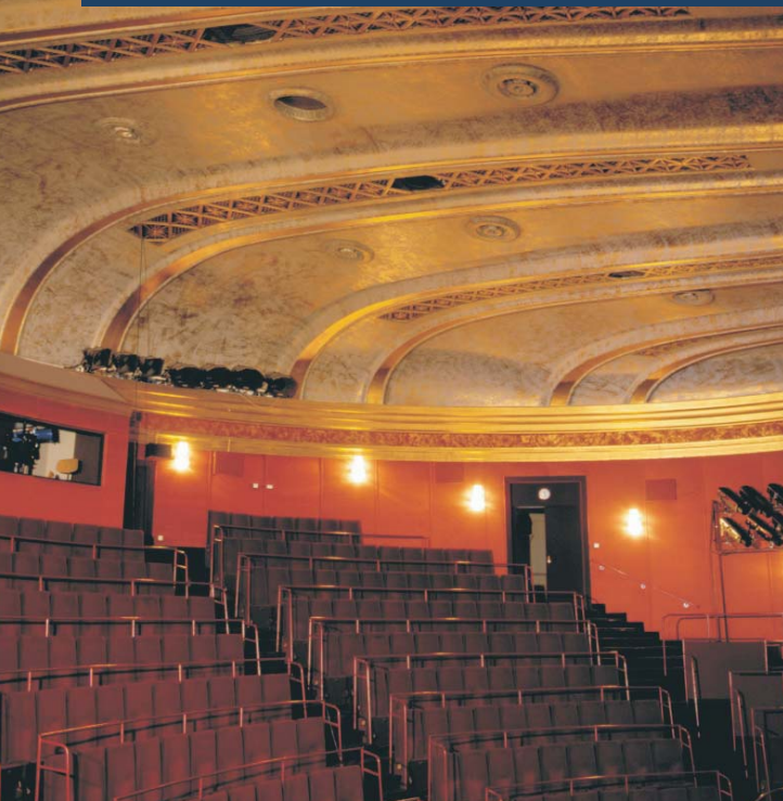
Variable twist outlet with core tube, type DD-VK, in the ceiling of 'Raimund Theater', Vienna / A
