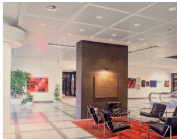
Twist outlet in the entrance hall of DEA Mineralöl AG, Hamburg / D
