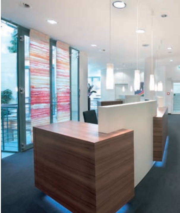
Radial outlet with circular face in a reception area
