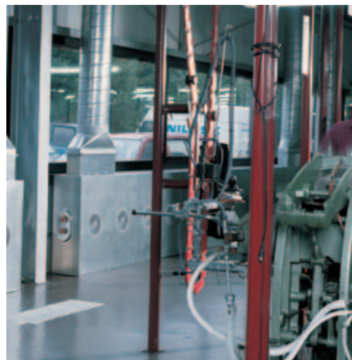
Figure 8: Air outlet in an ironing shop
