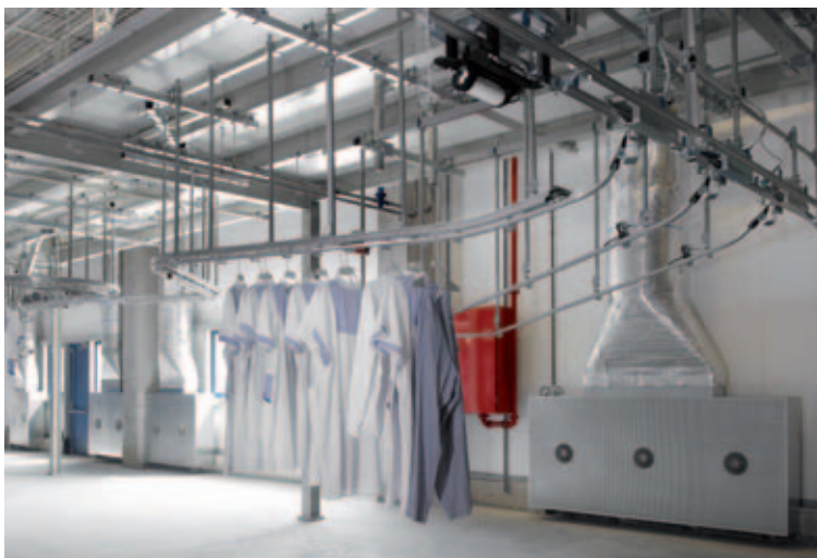
Figure 7: Air outlet in an industrial textile cleaning facility
