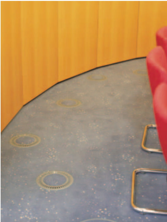
Fig. 3: Floor displacement outlet in a meeting room
