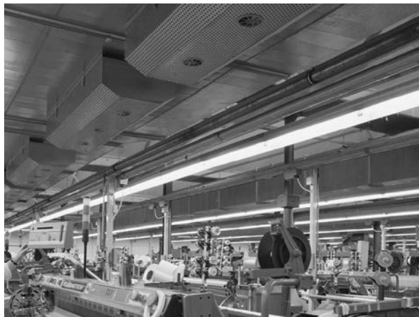
Figure 8: Trapezoidal displacement outlets below the supply air duct in a weaving mill
