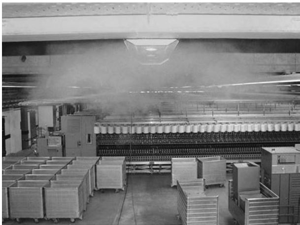
Figure 6: Trapezoidal displacement outlet - Jet dispersion made visible with smoke tracer
