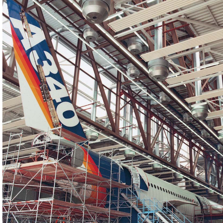
Conical displacement outlet, type VA-K, in the maintenance and painting hangar of 'Aircraft Services GmbH', Lemwerder / D
