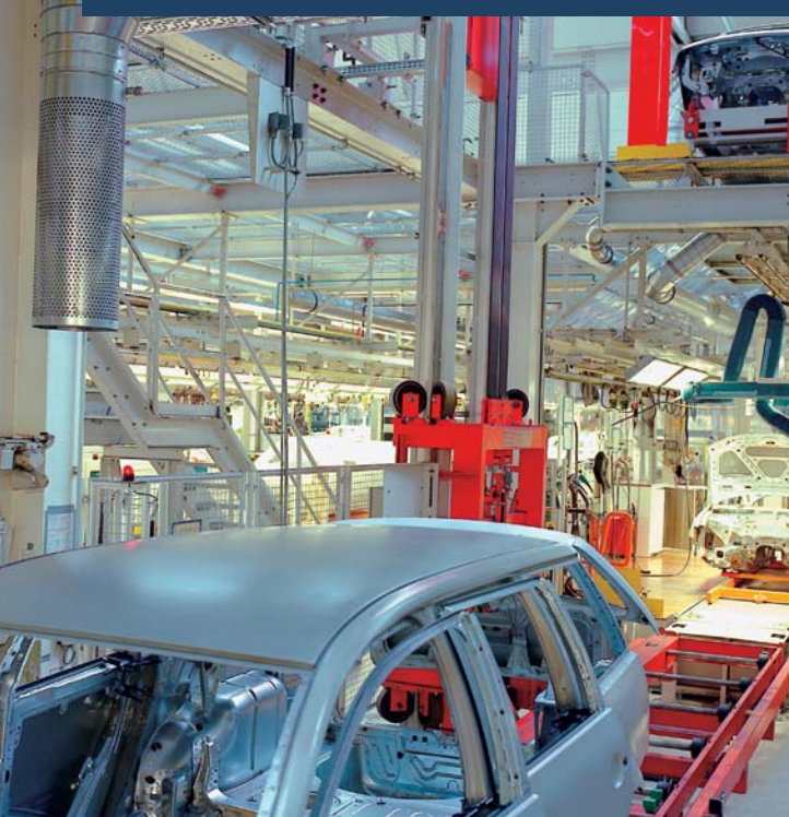
Circular displacement outlet, type VA-ZD, in a production hall of VW at Emden / D
