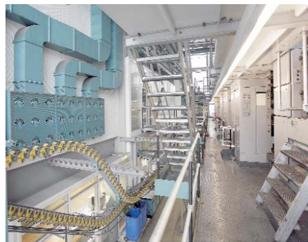
Rectangular displacement outlet, type VA-RN, in the printing shop of 'Vorarlberger Medienhaus', Schwarzach / A
