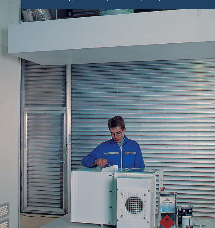
Laminar outlet, type VA-L, at a paint touch-up workplace
