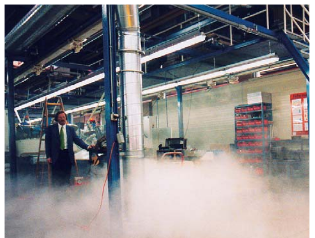
Circular displacement outlet, type VA-ZD, on the floor of the production hall of 'Stihl & Co.' at Wil / CH
