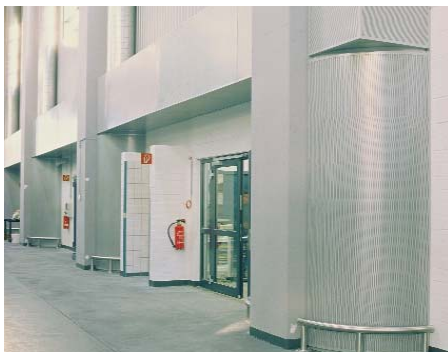
Rectangular displacement outlet and displacement quadrant in the Axel Springer publishing house, Essen-Kettwig / D
