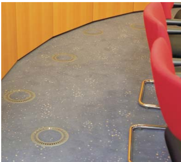
Floor displacement outlet, type Q-B-DN 215, in a meeting room at Lotto Rheinland-Pfalz, Koblenz / D
