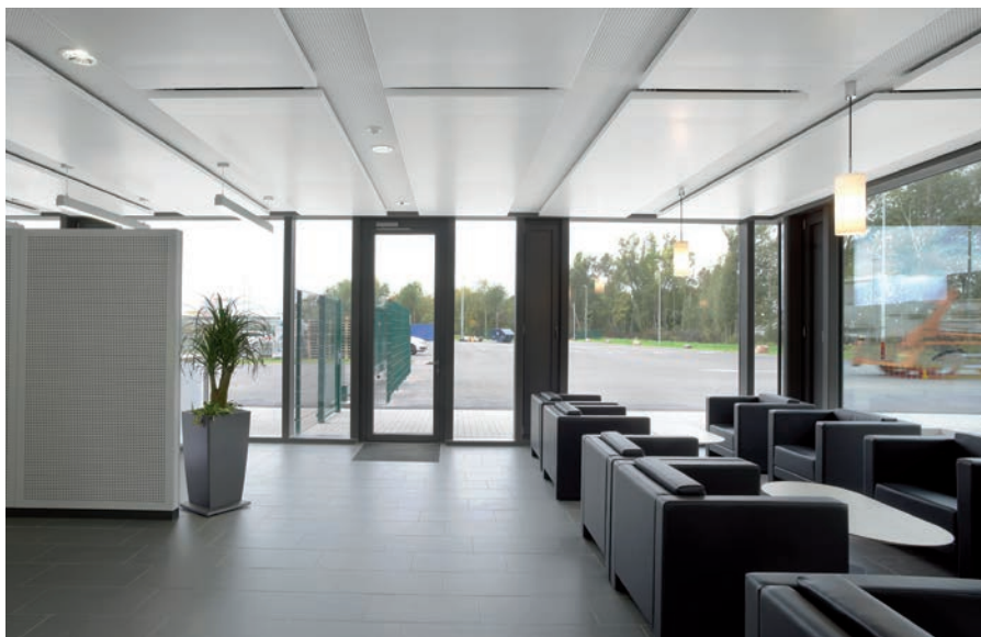
Chilled sail AVACS
