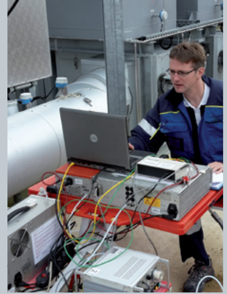
Functional testing at a thermal incineration plant
