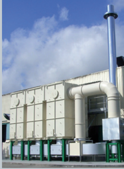
Post-combustion plant with heat recovery for emissions reduction
